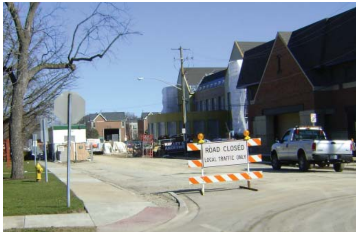
Looking east on Prairie from Washington. While the new library goes up, the Village is converting Prairie into a cul-de-sac to improve safety and access to the new building.
