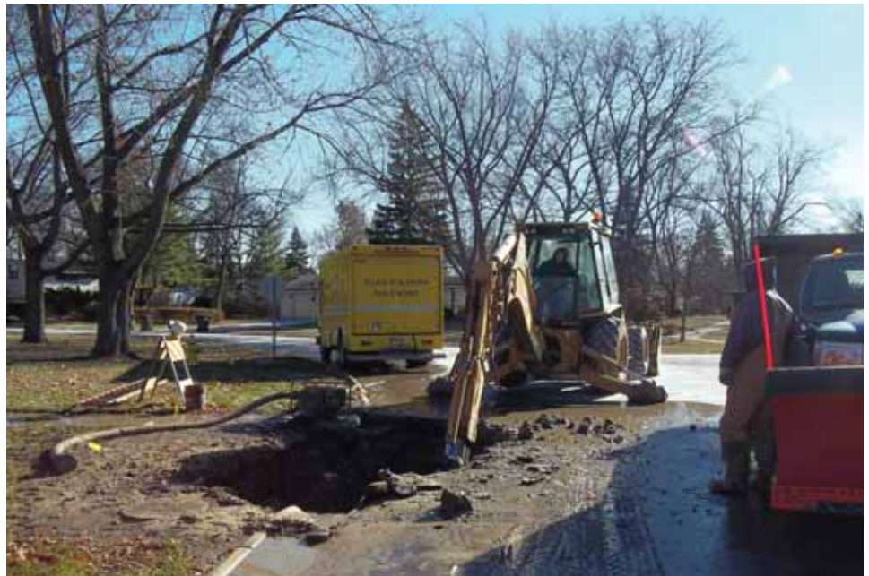
Public works crews repair a water main break by first excavating to expose the damaged pipe.
