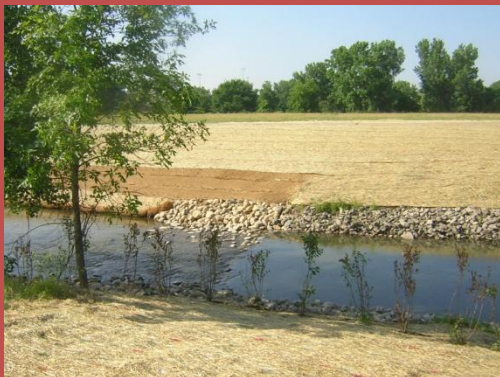
Top: Slumping streambank at Lot 16 Bottom: Restoration construction in progress
