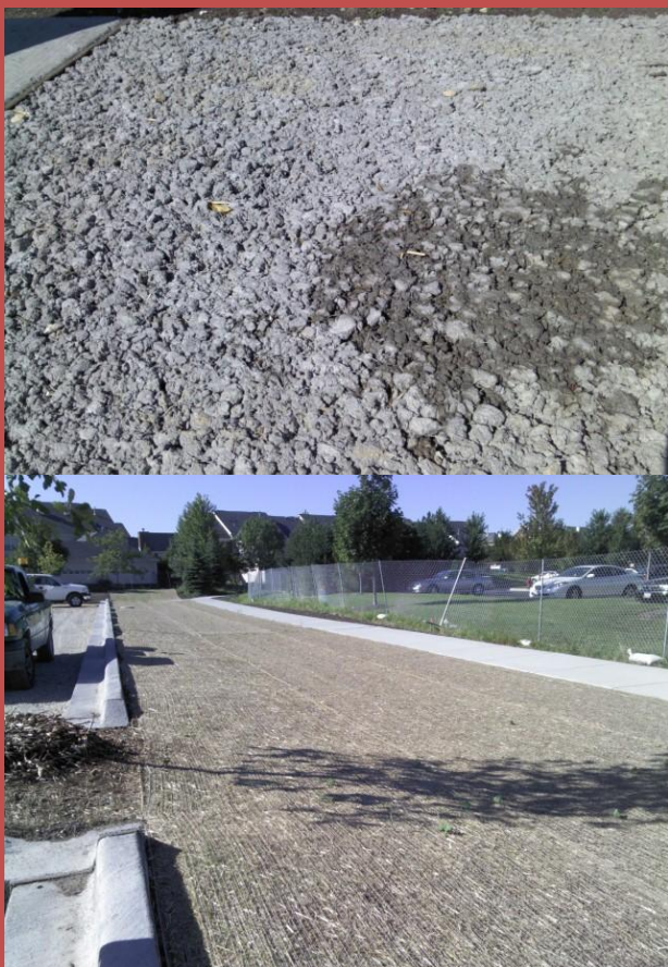
Above: Close-up of pervious concrete at the site Below: Bioswale before vegetation
