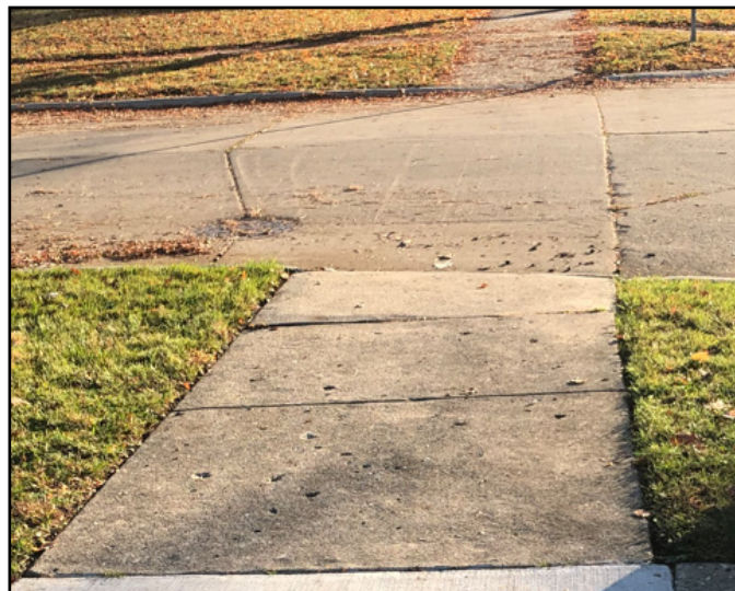
EXHIBIT 2: CURB RAMP WITHOUT DETECTABLE WARNING STRIP
