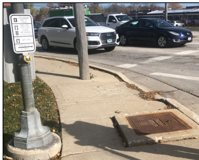
EXHIBIT 3: CURB RAMP WITH NON-COMPLIANT TURNING SPACE AND GUTTER TRANSITION
