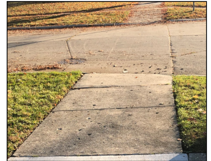
EXHIBIT 2: CURB RAMP WITHOUT DETECTABLE WARNING STRIP
