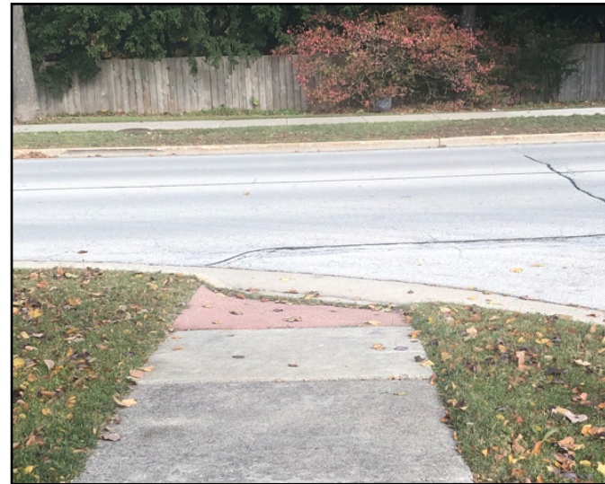
EXHIBIT 4: MISSING RECEIVING CURB RAMP
