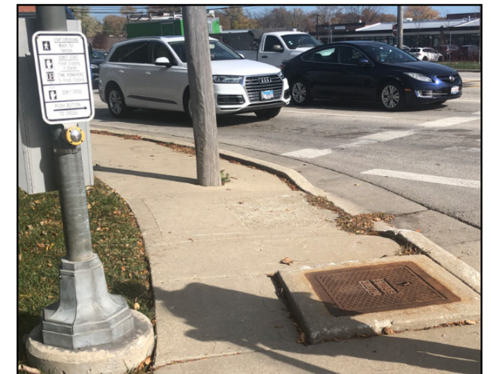
EXHIBIT 3: CURB RAMP WITH NON-COMPLIANT TURNING SPACE AND GUTTER TRANSITION
