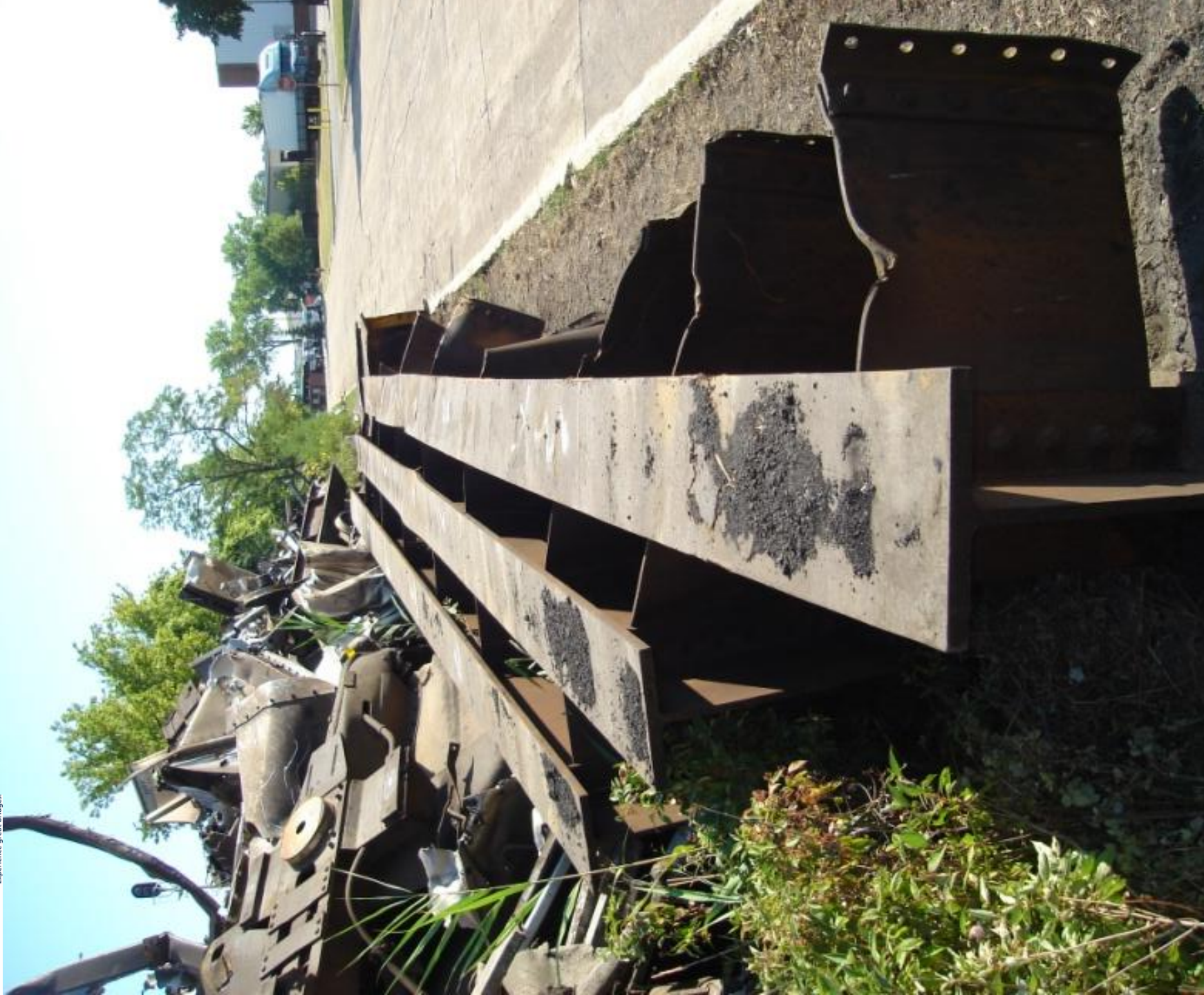
Beam Set 2 – Beam material found in full section. All “dings” are new.
