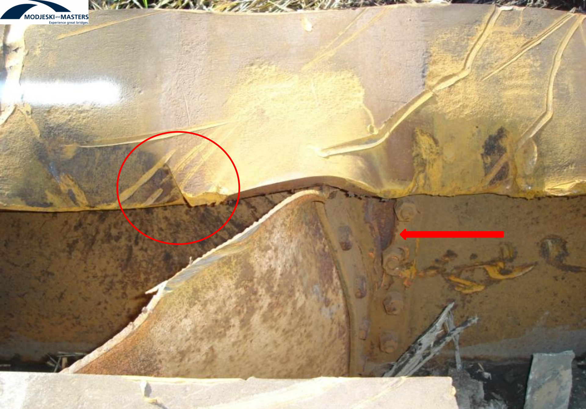
Beam Set 1 – Tear in flange with fresh rust indicating accident damage (circle); Diaphragm connection angle torn in accident (arrow)
